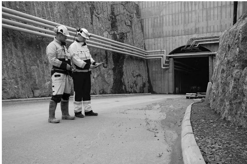
Figure 16.3 Construction of an underground repository for spent nuclear fuel in Finland. Source: Posiva Oy, http://www.posiva.fi/ .
